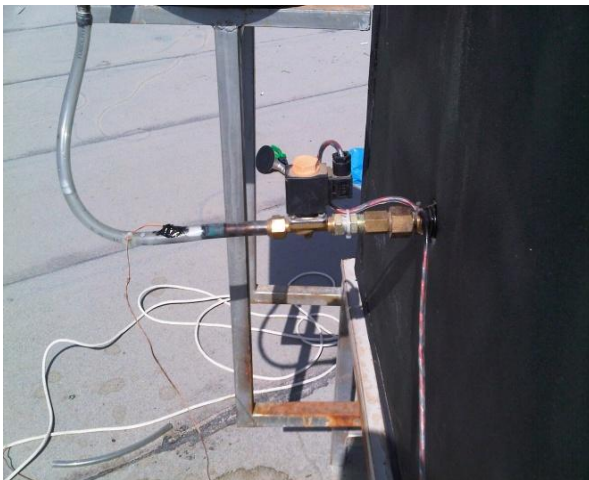
Fig.3. Solenoid valve for water level control
